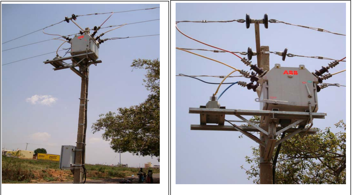
Photographs showing the Mounting details of Auto reclosures on single pole (RCC square type) for 11 KV feeders at project site
